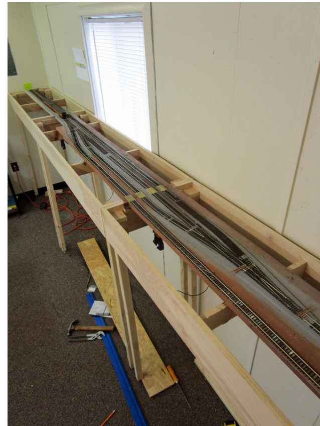
10. Laying the track, installing the turnouts, and attaching feeder drops to the rails.
