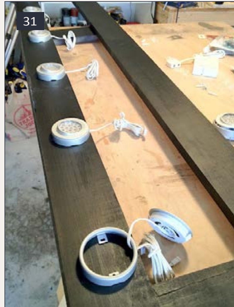
31: I installed two packs of Ikea "Inreda" LED pucks along the underside of the valence framework. They put out no heat whatsoever (which is good, since my garage already gets over 100 degrees F in the summer) and can rotate / adjust some to direct the light.
