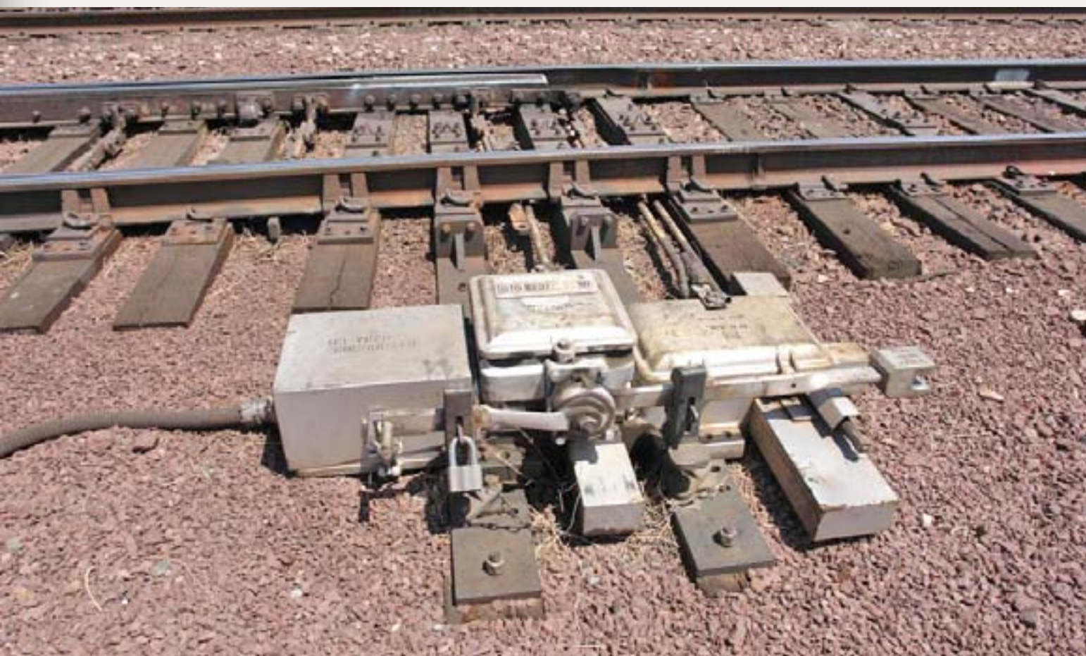
Figure 9. West Goffs remote switch.
