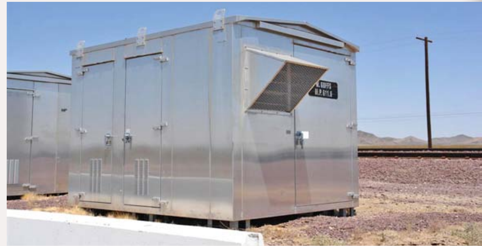
Figure 2. West and south sides of the generator cabinet.
