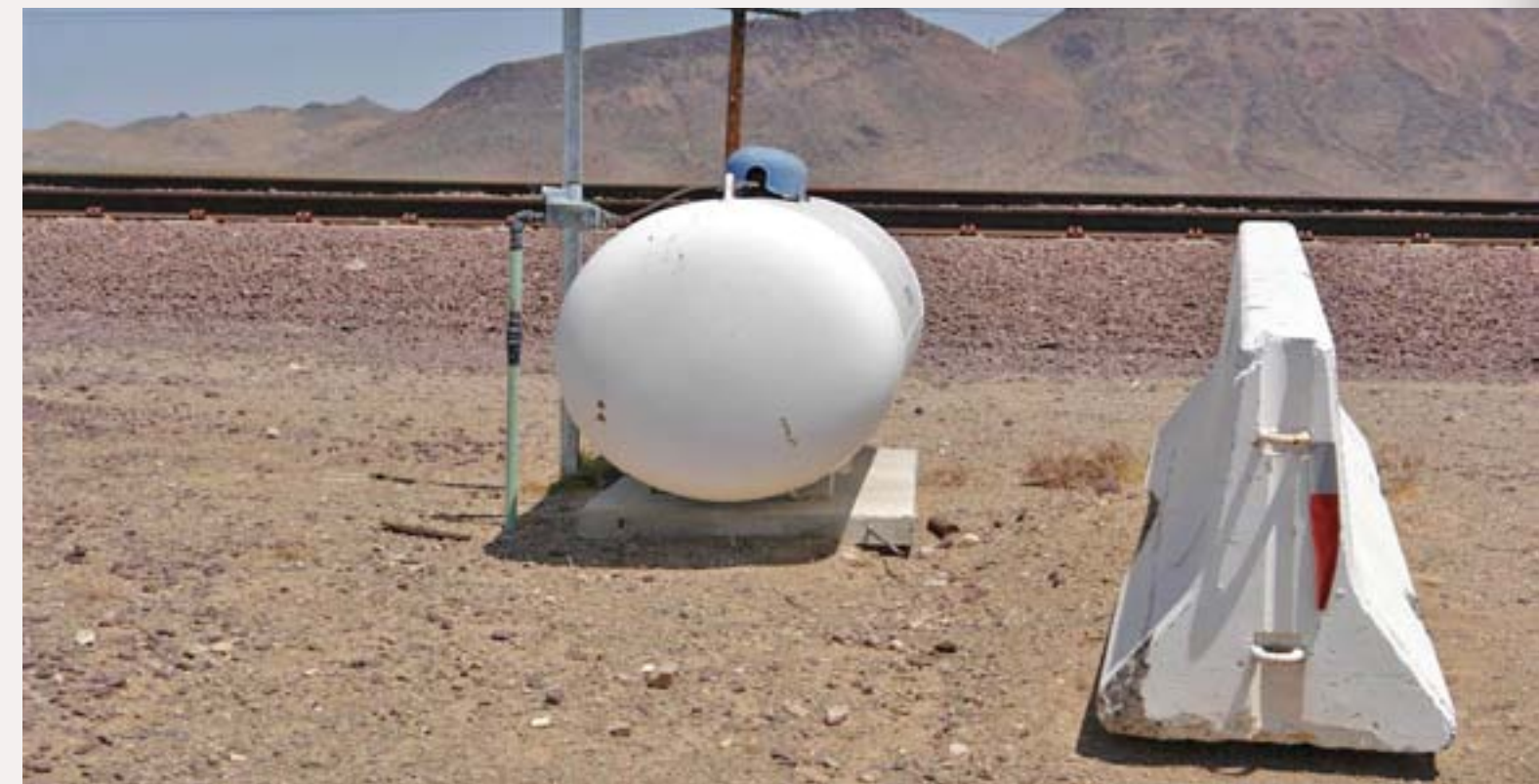
Figure 3. Propane tank and jersey barrier.
