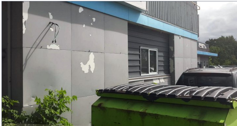
14. Sometimes accidents are happy ones! Some of the paint was removed with the masking tape, but it simulated the peeling paint on the actual building.
